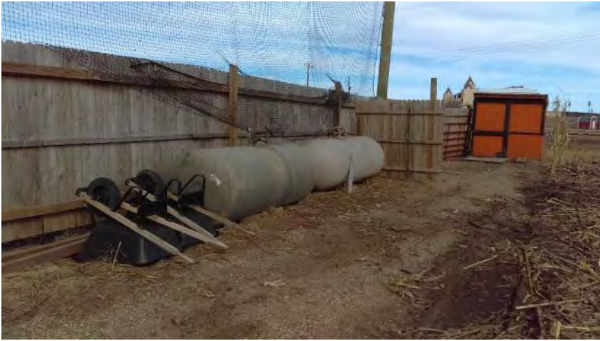
9) Propane tanks associates with Sever's buildings
